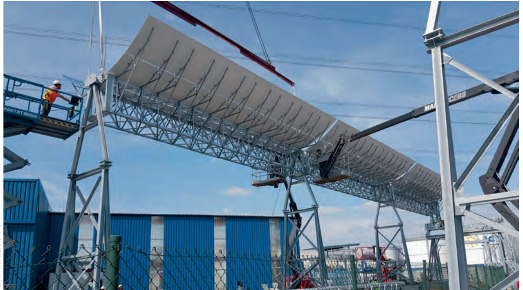
Concentrated solar thermal pilot plant in Antwerp
