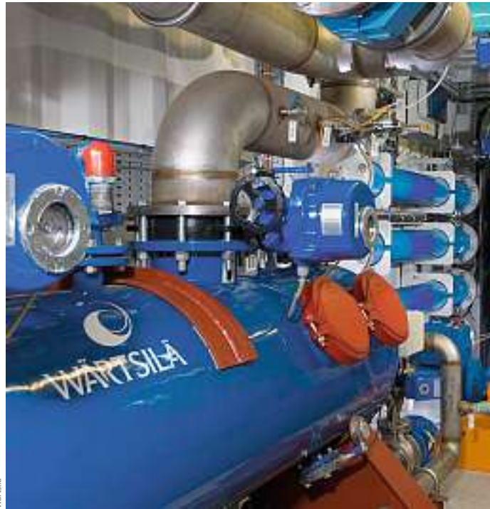
Wärtsilä's Aquarius EC Ballast Water Management System. The United States has yet to approve a BWMS system.
