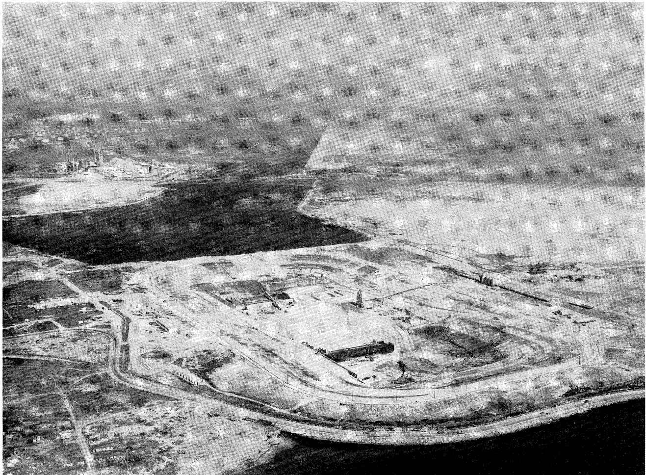
7. The building site of the large lock which will be accessible to bulk carriers of 200,000 tons as from 1971.
